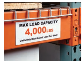
T4: Beam Load Capacity Label
